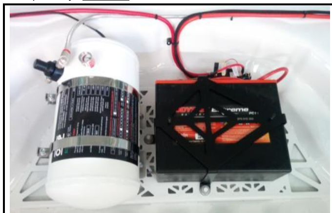
E1-2) Battery – in location
