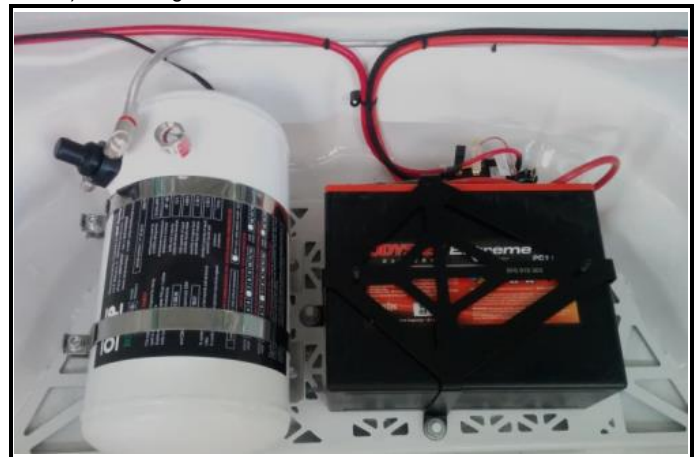
S4-2) Fire extinguisher in location
