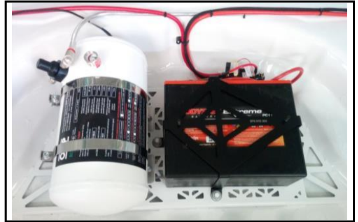
E1-2) Battery – in location
